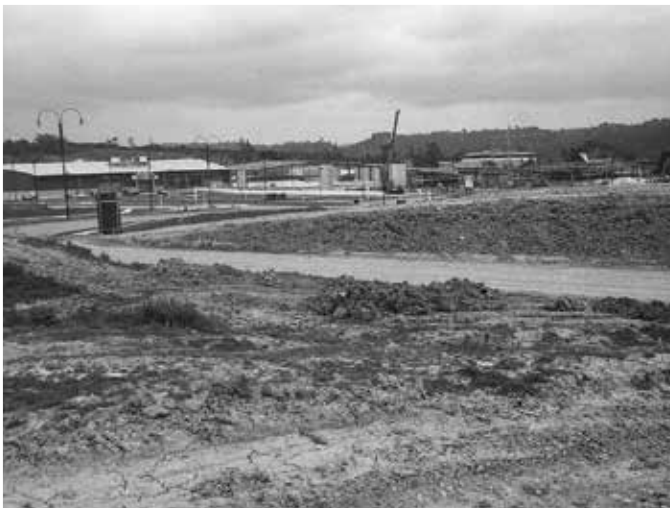
Don McKinnon Drive under construction. Old PlaceMakers on the left, University right distance.
