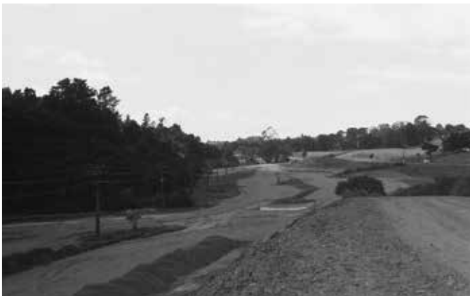
Constructing the present Oteha Valley Road. The old road is centre right
